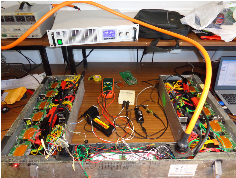
(b) Charging test. Special connector emulates a number of the car's systems. LED (bottom left) indicates high voltage.
